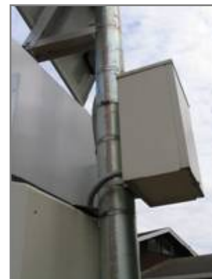
Pole-mounted battery box
